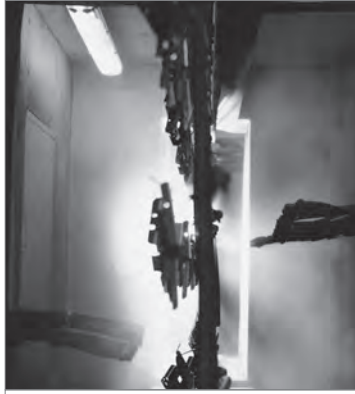
Robotik Boya Tesisi Robotics Paint Facility
